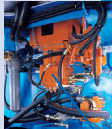
Hydraulic unit driven by an AC motor
