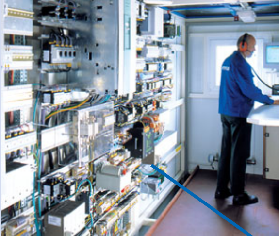
Air-conditioned electrics compartment
